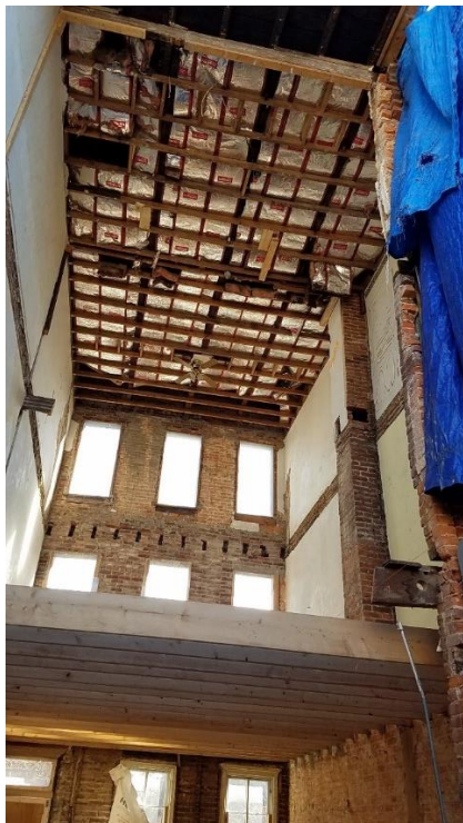
Image 6: 1426 Hollins Street – Existing conditions at first, second and third floor looking toward front façade and remaining roof and side walls, March 12, 2021
